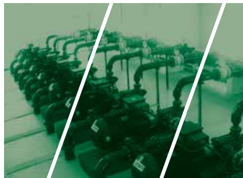
Boosting and Distribution of surface water
